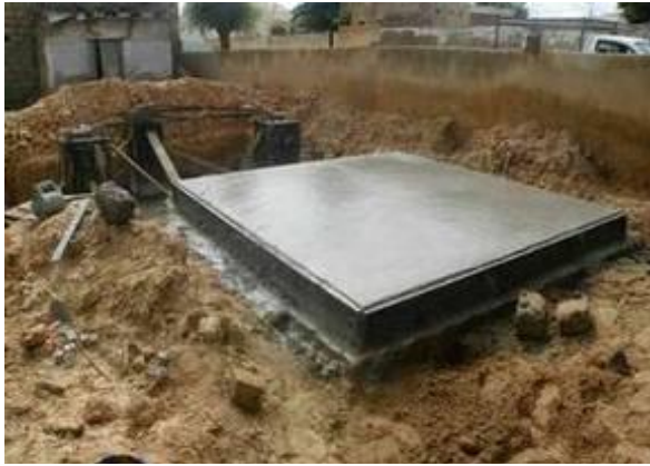
Figure II.7: Plateforme du Shelter.
