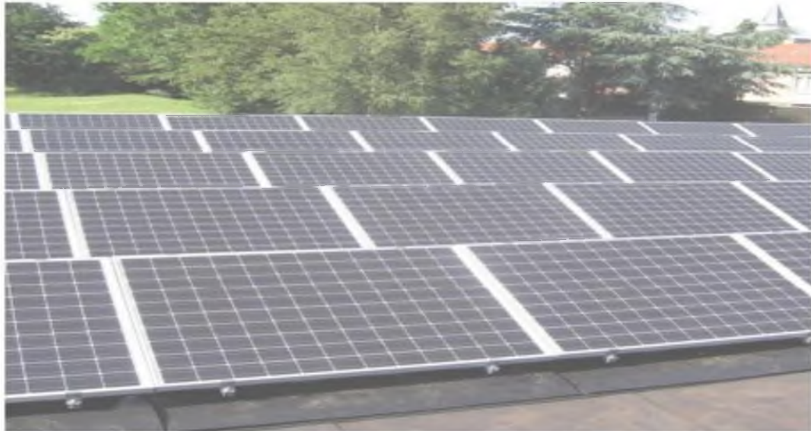
Figure 3.2 Installation photovoltaïque autonome
