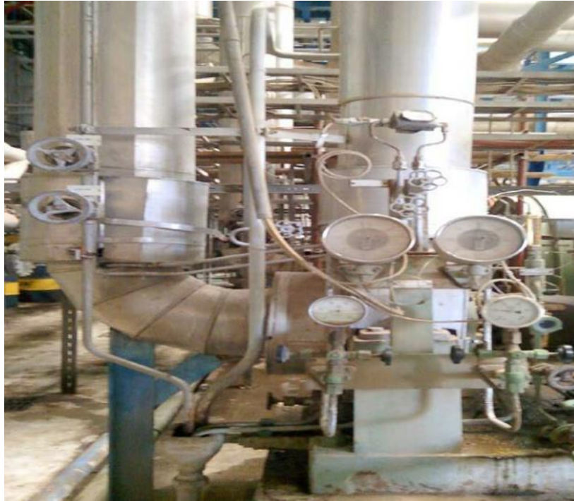
Figure II.3: photo la pompe nourricière
