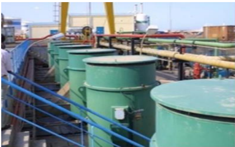
Figure I.14 : station de pompage
