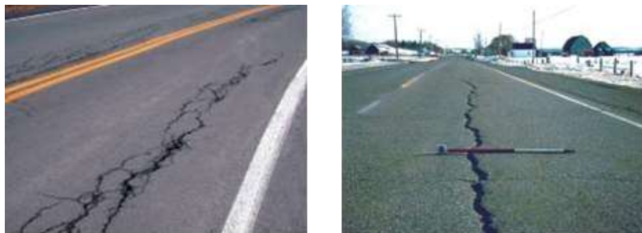
Figure I.17 : Fissuration longitudinale. (MDCS, Québec ,2002)
