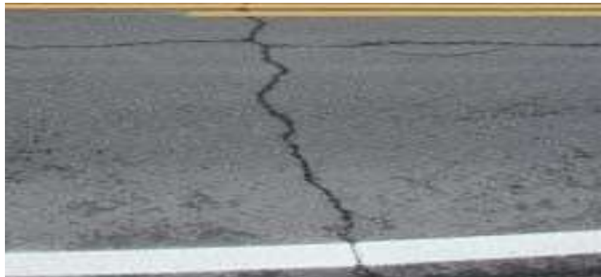
Figure I.16: Fissures transversales. (MDCS, Québec ,2002)
