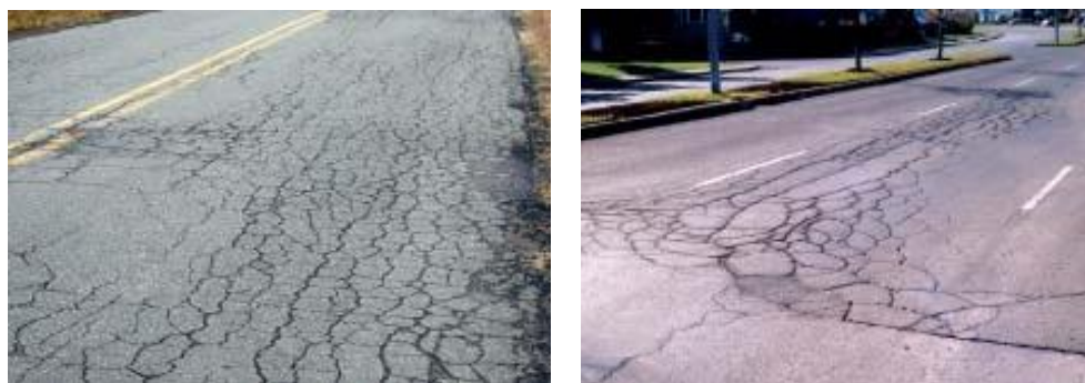
Figure I.21: Faïençage.(Fissures en carrelage)
