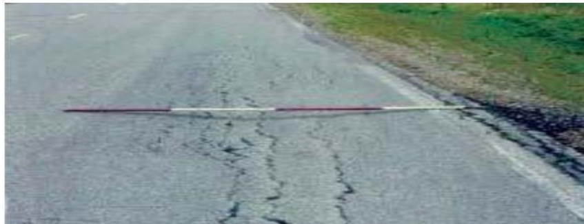
Figure I.16. Affaissement hors rive (LCPC, 1998)
