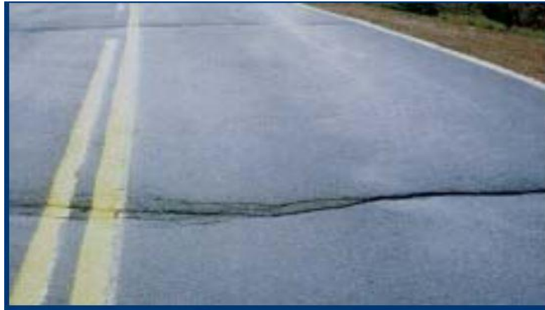
Figure I.19. Fissures transversales (MTQ, 2002)
