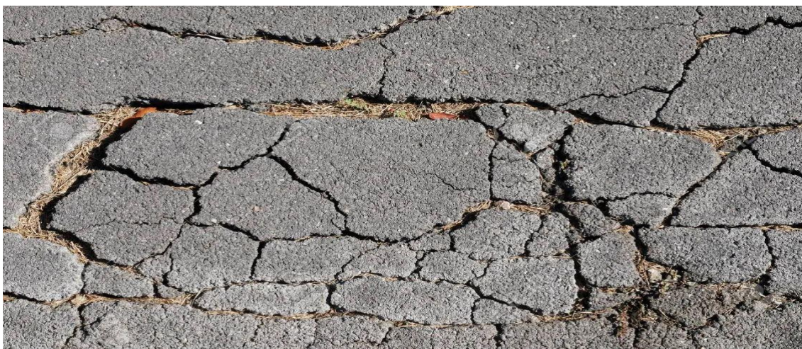
Figure I.20. Le faïençage (Btpnews, 2022)
