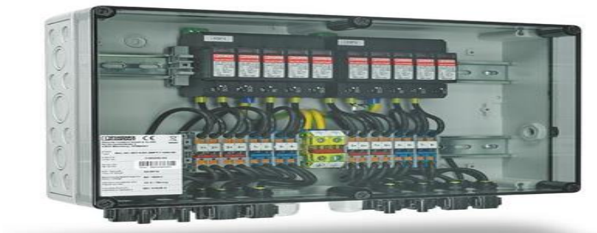
Figure II.6 : Coffret de raccordement
