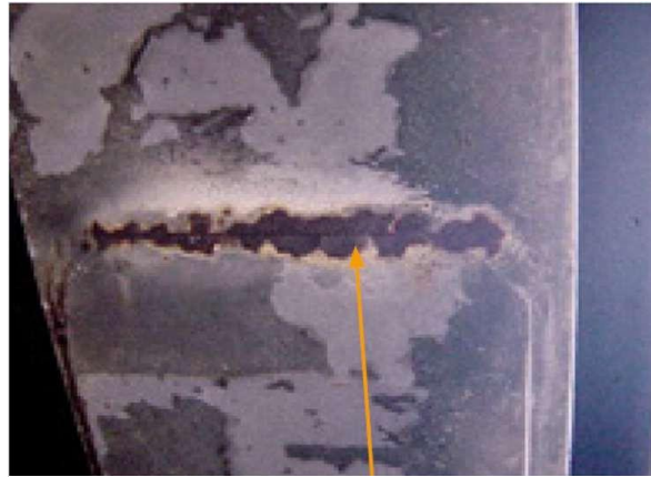
Figure I.2 : Fissure de fatigue [3]
