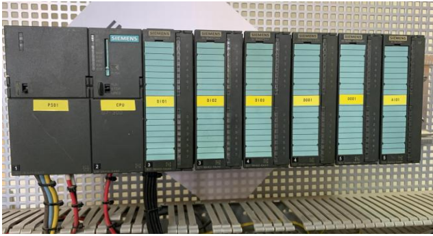
Figure III.2: API Siemens s7-300.
