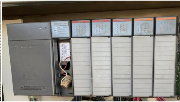
Figure III.3: API Allen Bradley SLC500.
