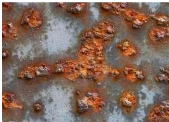
Figure I.6 Corrosion inter granulaire
