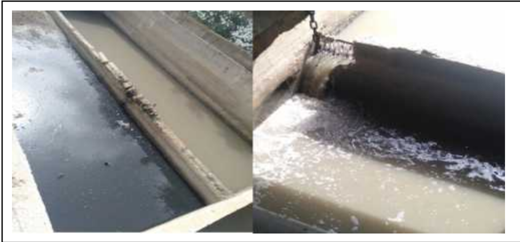
Figure04: Station de relevage N°1.
