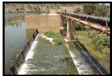
figure38:La station de pompage de lac de Reghaia source: www.google.com
