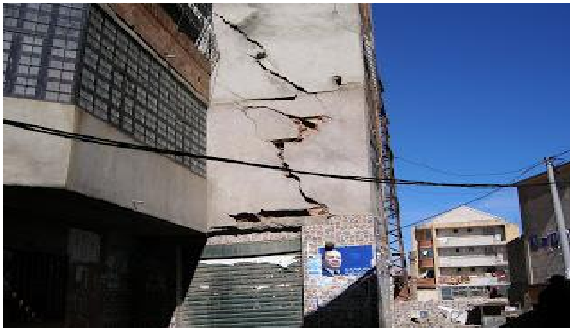
Figure n°6.II : Fissuration des constructions.
