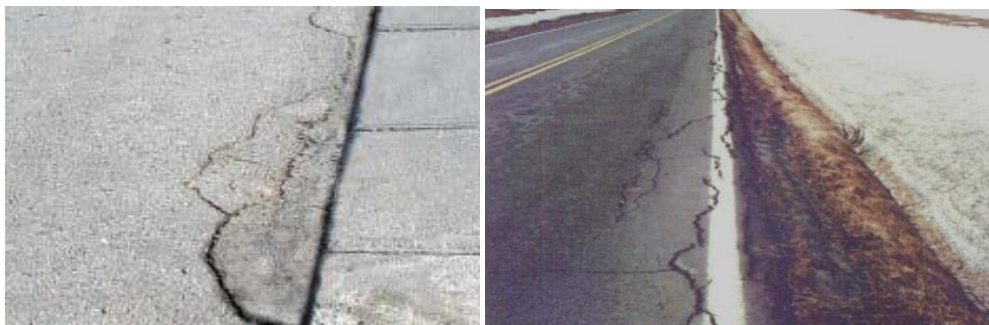
Figure I.30 : Fissures de rives.
