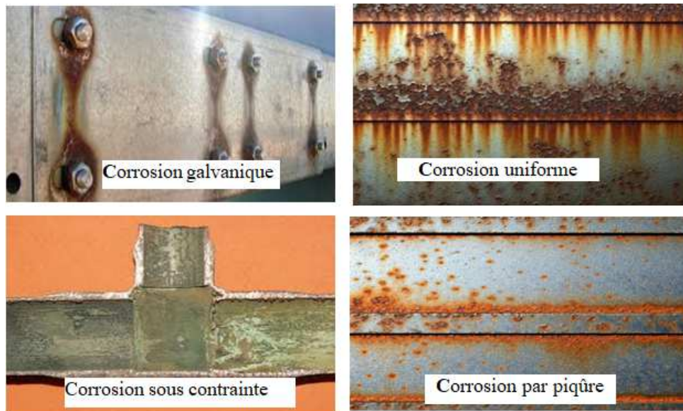
Figure I.1 : Types de Corrosion.
