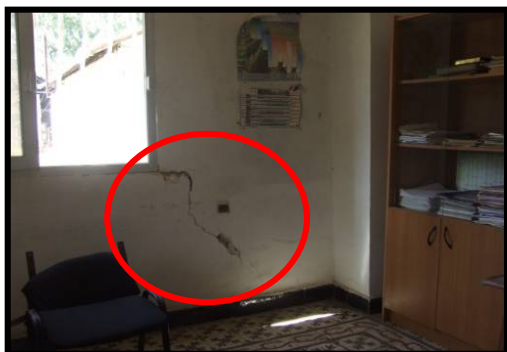
Photo 4.93: Fissure diagonale importante
