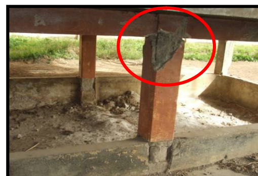
Photo 4.104: Corrosion des poteaux
