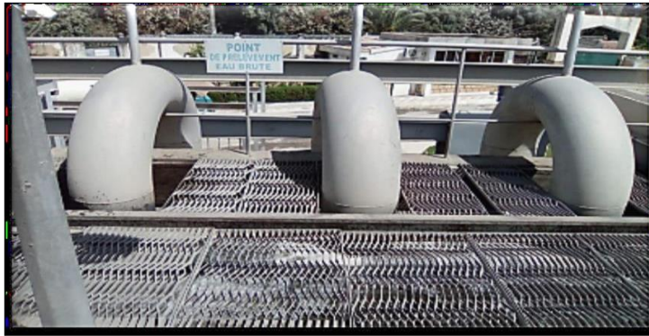
Figure 7. Poste de relevage (ONA, 2022)
