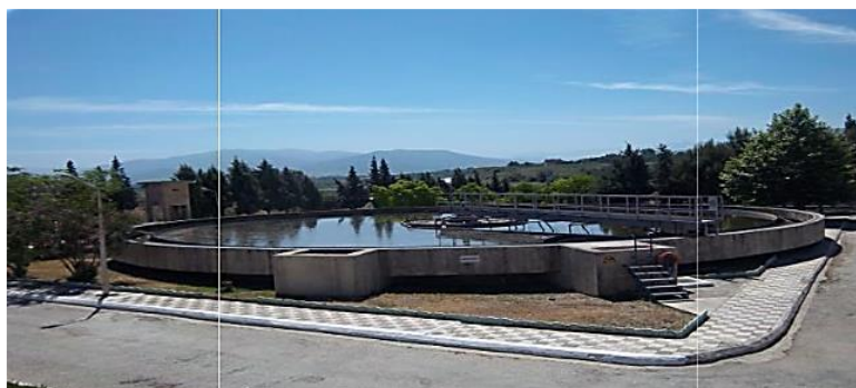
Figure 12. Bassin de clarification fin (ONA,2022)
