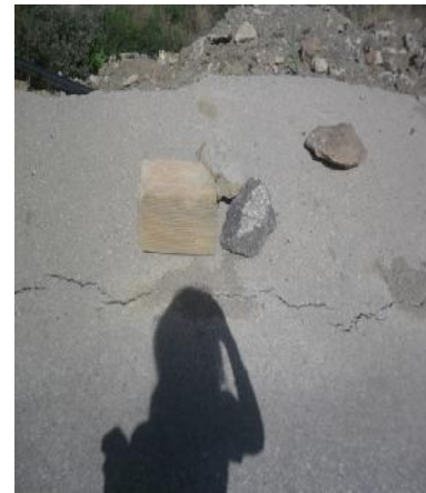
Fig III.13-8: Fissuration de CW. (CHERGUI.2016)
