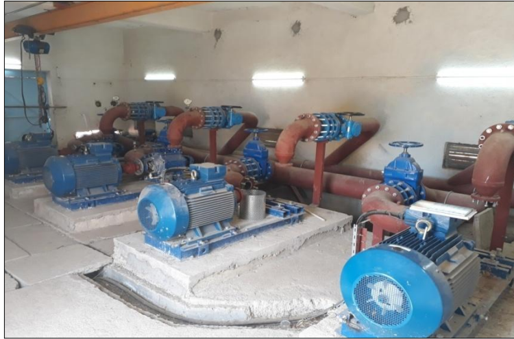
Figure (II .8): Station de pompage Tassifth Ait Khellili SP 1
