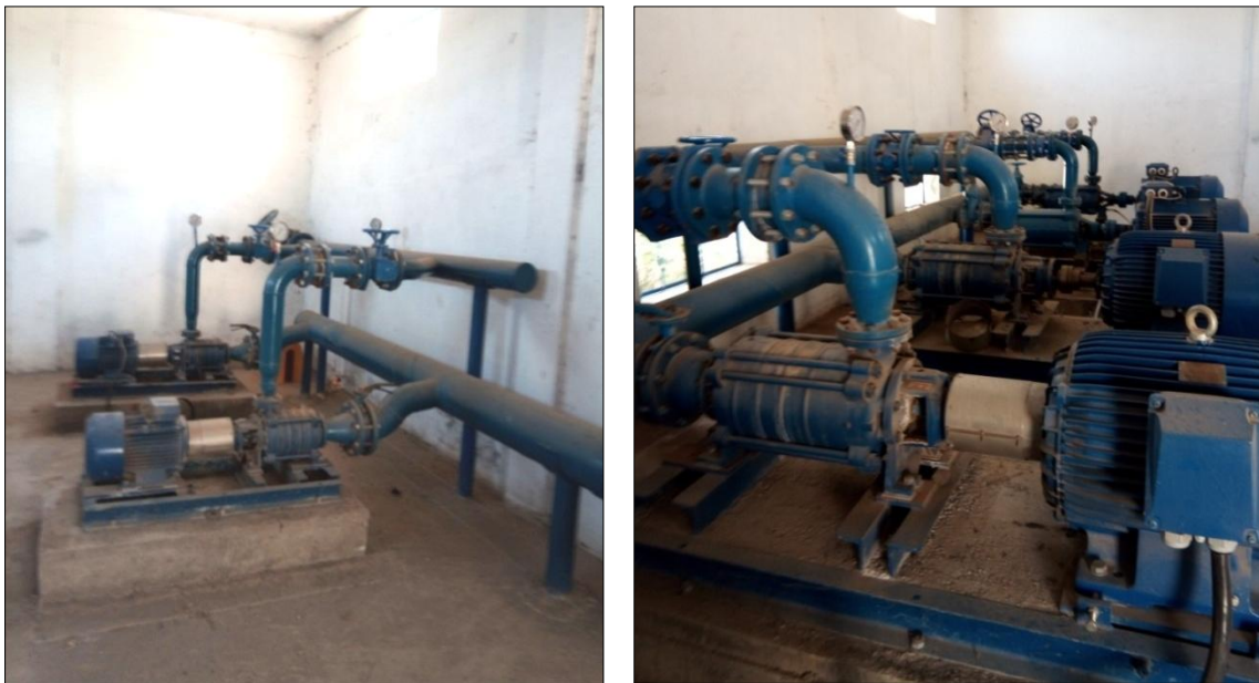
Figure (II.11): Station de pompage Ilmatene (Ait Zellal) SRI
