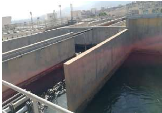
Figure III.5: Chambre de mélange
