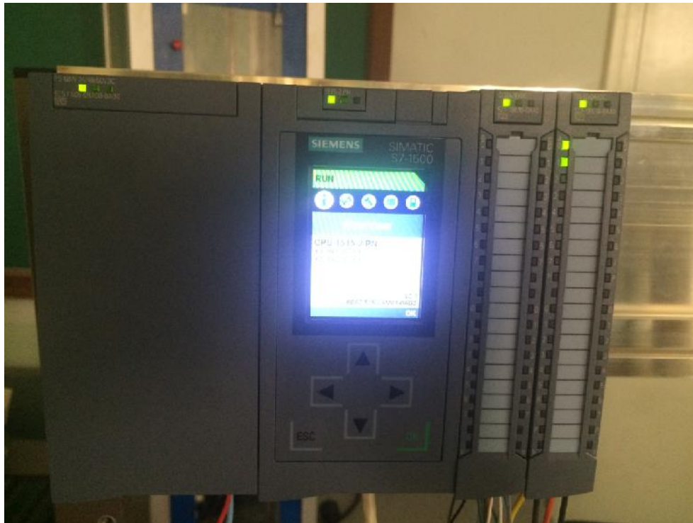
Figure 3.1: L'automate SIMATIC S71500
