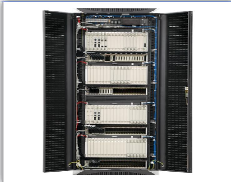
Figure III.4 : L'armoire du MSAN indoor. [21]
