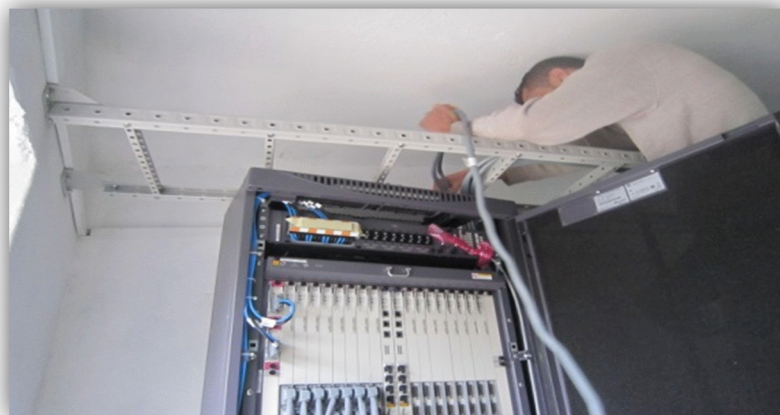
Figure IV.8: Raccordement des câbles.
