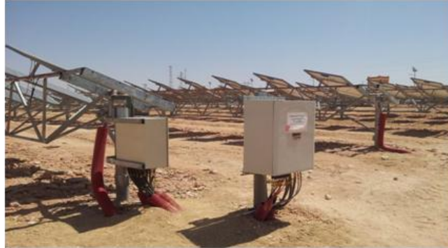
Figure III.8 : Boîte de raccordement
