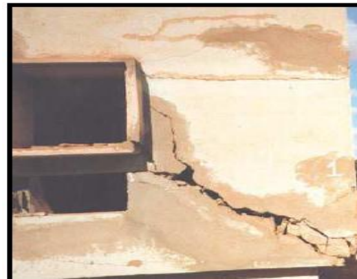
Figure II.2 : Fissures diagonales (Derriche Z et al.2002 )
