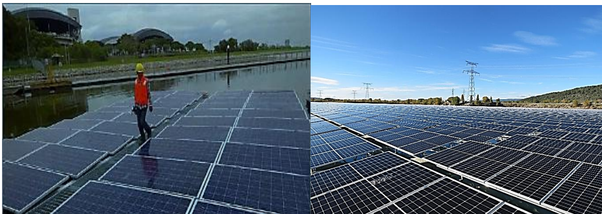
Figure.II.1. Installations photovoltaïques flottantes [4] [21].
