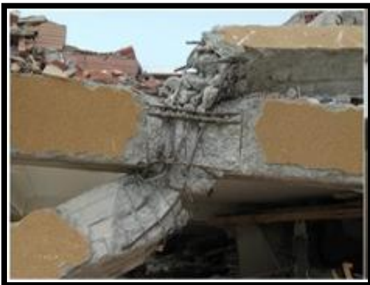
Figure .I 15 Rupture en zone nodale section ( Davidovici 2003)
