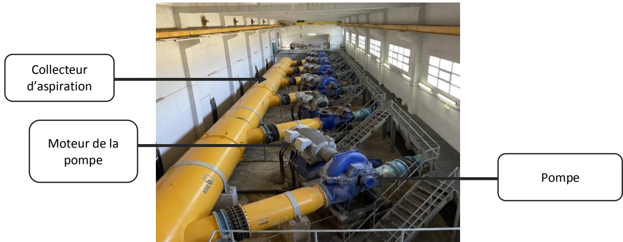
Figure I-4 : Station de pompage
