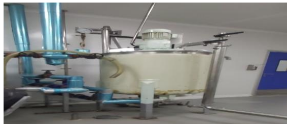
Figure III.13: Cuve de stockage
