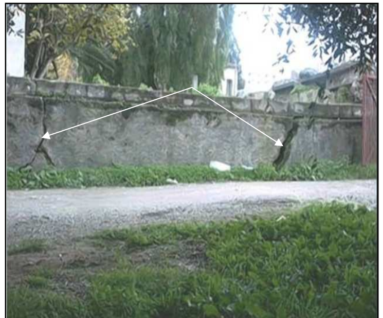
Fissuration du mur [11]
