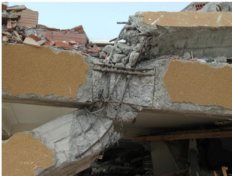
Figure I-14 Rupture de la zone nodale [1].
