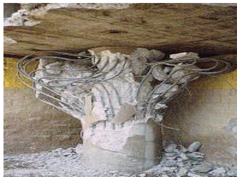
Figure I.6 : rupture de poteau (insuffisance de renfort transversal)
