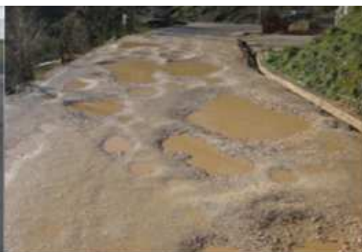
Figure II.23 : Dégradation de la route RN15, village Soumer.
