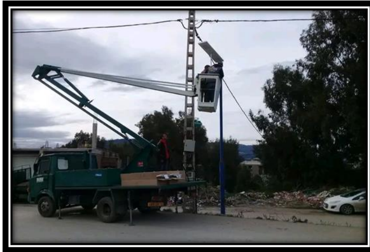
Figure 19: installations d'éclairages publics
