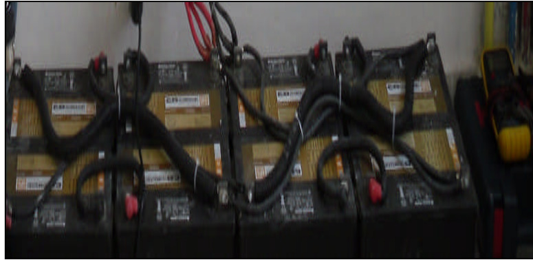
Figure I.13 : Batteries de stockage
