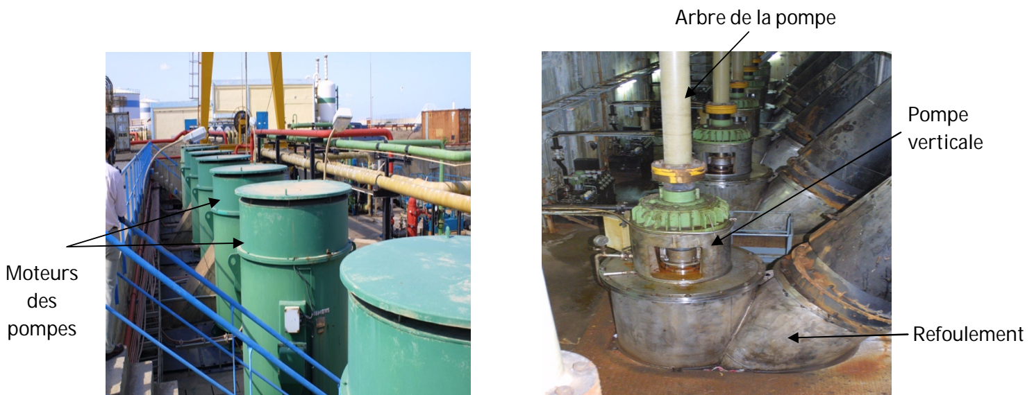
Figure I.2 : Station de pompage
