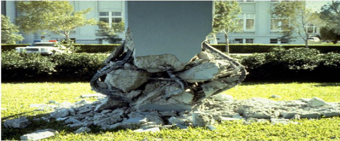
Figure II.22: Non confinement du béton [10]
