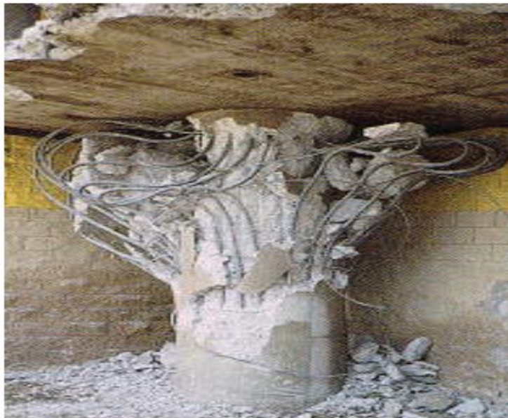
Figure I.4 : Rupture de poteau (insuffisance de renfort transversal) [23].
