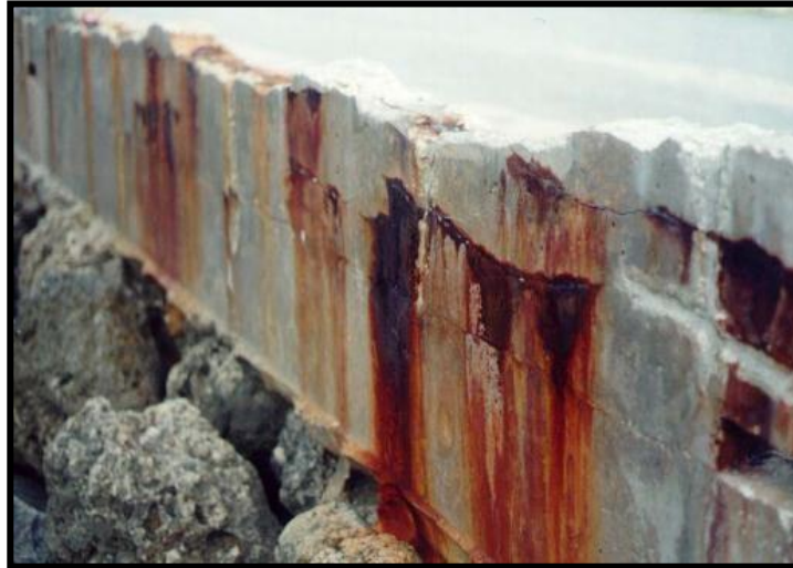
Figure I.1-4 : Corrosion des armatures [8]
