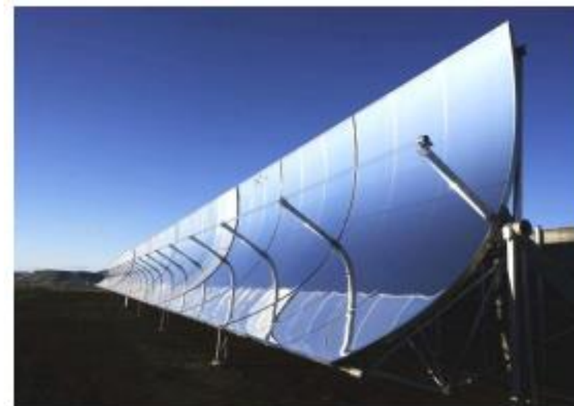
Figure II.8 : Photo de la centrale CSP Nevada Solar One[20]
