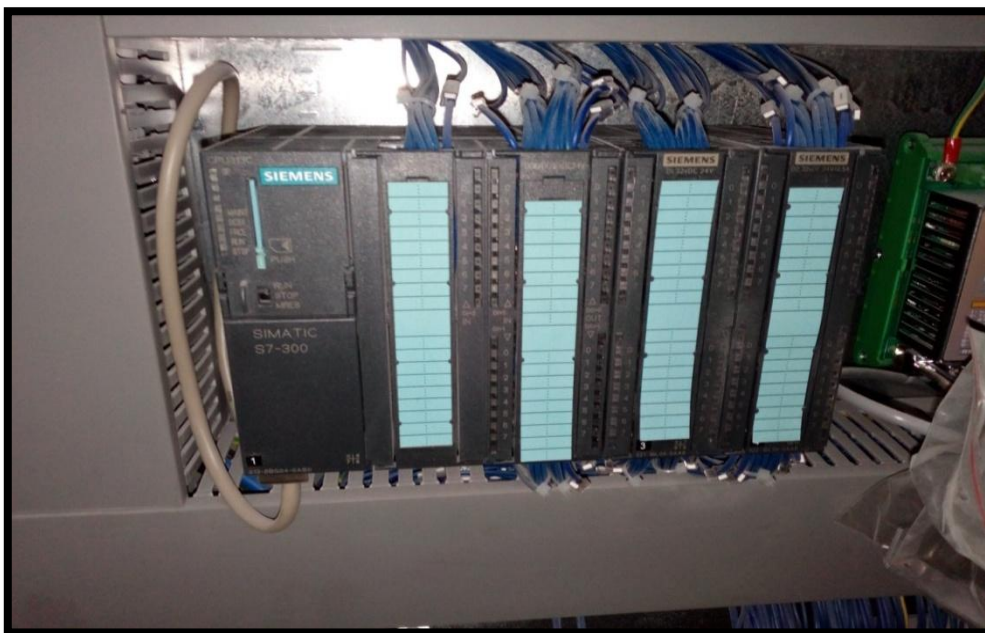
Figure III.1. Automate S7300 SIEMENS.
