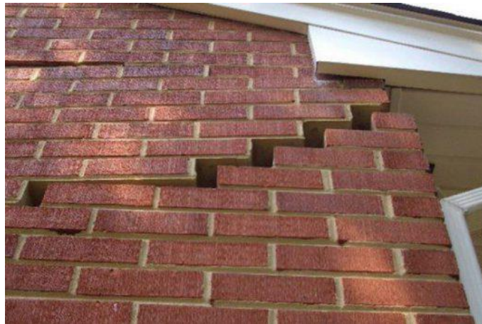
Figure 1.8. Fissures dues aux tassements.
