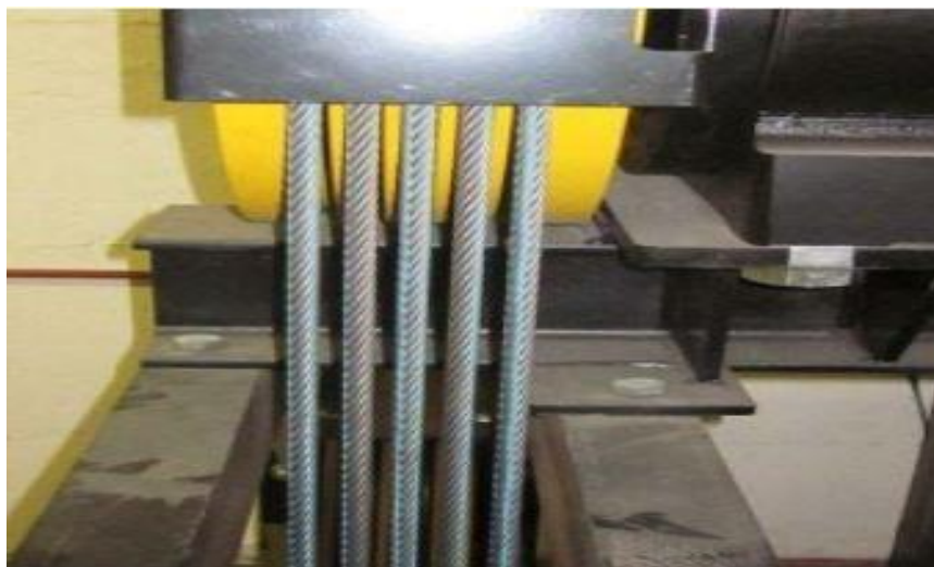
Figure I.22: Câbles de traction.
