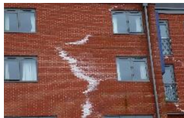
Fig. II. 8 : Efflorescence. Source: The Camberley Society
