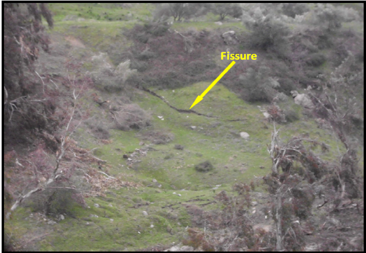
Fig. III.30: Fissuration du sol
