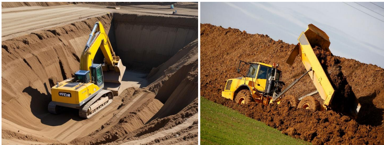
Figure V.4. Examples of embankment and excavation. Source: Congo soutainement & Habitat Presto https://congousoutenement.com/ & https://www.habitatpresto.com/
