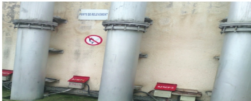
Figure 11 : Pompes de relevage (ONA)
