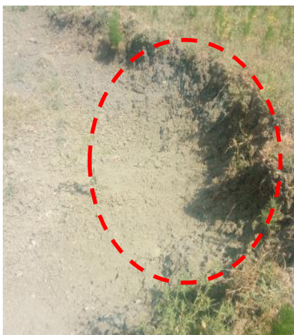
Figure 1.11 Erosion interne du talus aval
