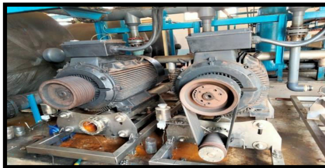
Figure III.14: Pompes à haute pression.
