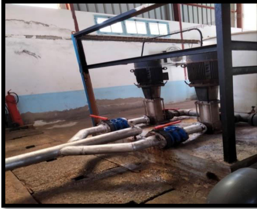
Figure III.17: Les pompes centrifuges
