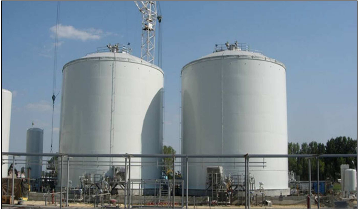
Figure I.3.9. Bacs de stockage.
