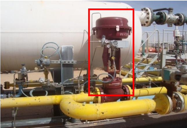
Figure III.7 : La vanne PCV-11208.
