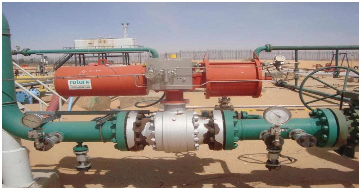
Figure III-9 : La vanne ESD-12000.
